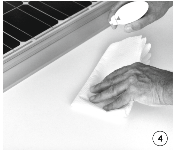
Use a degreasing agent to clean the motorhome roof and glue the spoiler on it. Let the glue dry.
